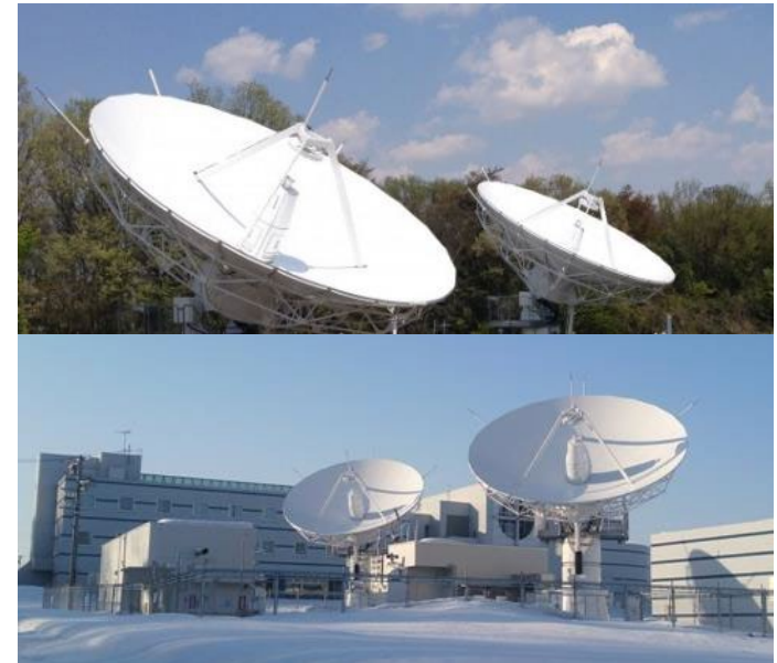
A group of antennas of the private company (at the main station and the sub-station)
