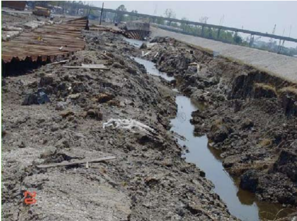
Figure 7.9 Industrial Canal East Bank South Failed I-wall
