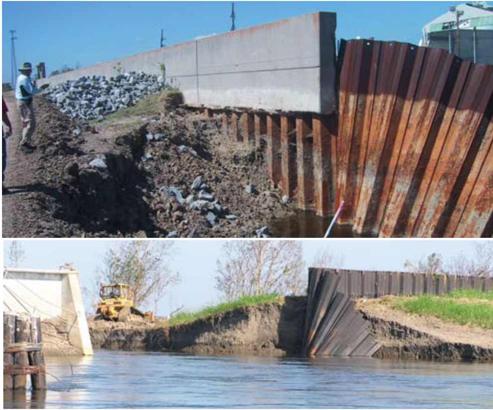
Figure 8.3 Failed I-Wall and Levee Sections
