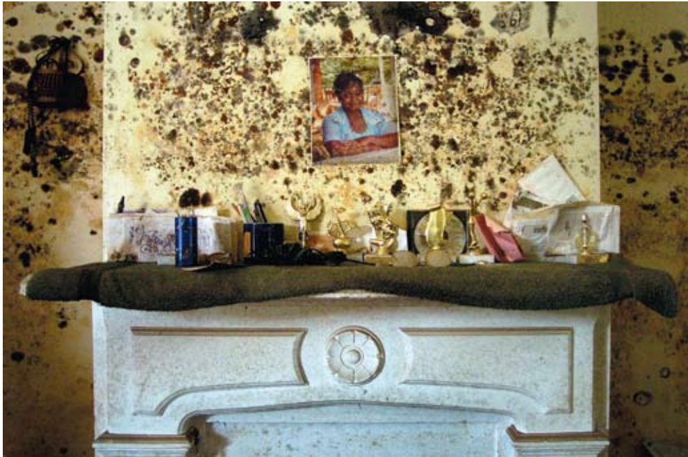
Figure 6.10 Overrun by Mold
