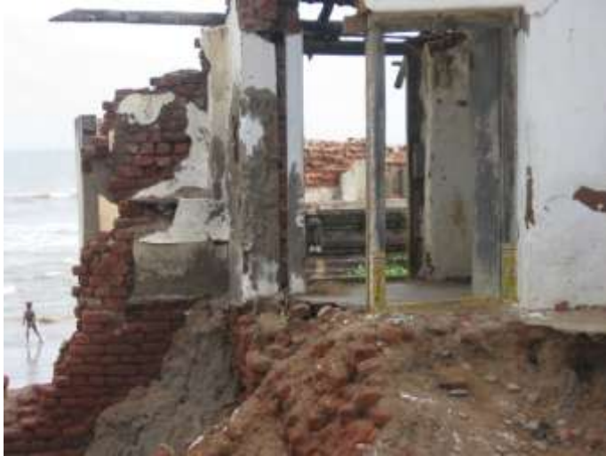
EFFECT OF BEACH EROSION IN UPPADA VILLAGE
